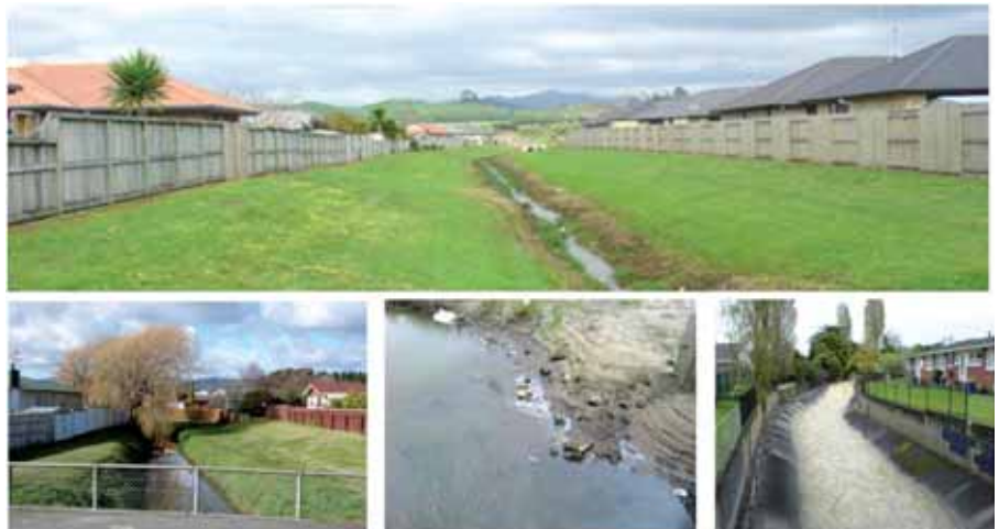
Examples of 'conventional' responses to blue network issues at the local level. These often poorly relate with their settings, creating risks for flash flooding, lower property values and lowered safety levels.
